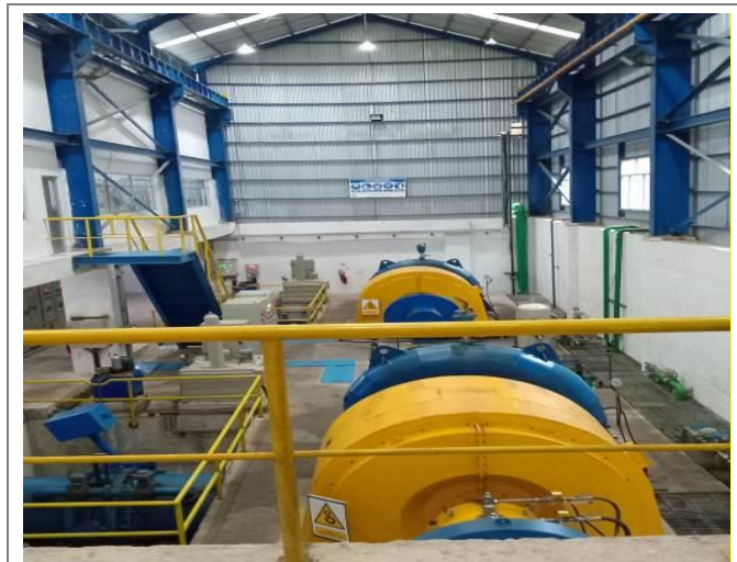
FIGURE 12: TURBINE GENERATOR AT PARMONANGAN 2 MINI-HYDRO PP
