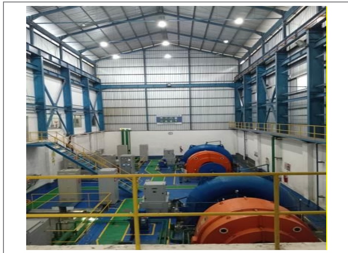
FIGURE 11: TURBINE GENERATOR AT PARMONANGAN 1 MINI-HYDRO PP
